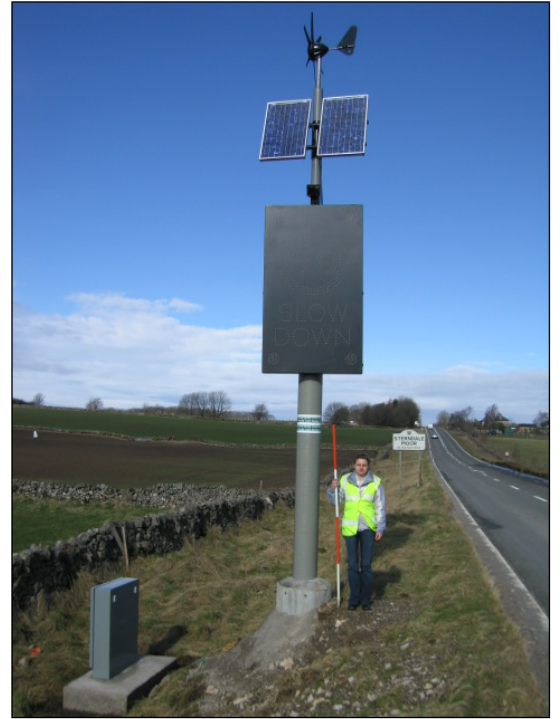
A515 - The only operational speed limit VAS with associated solar panels and wind turbine on this
