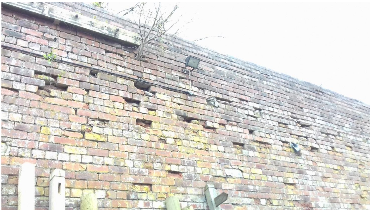
GOODS SHED INTERNAL ELEVATION SHOWING VEGETATION GROWTH
