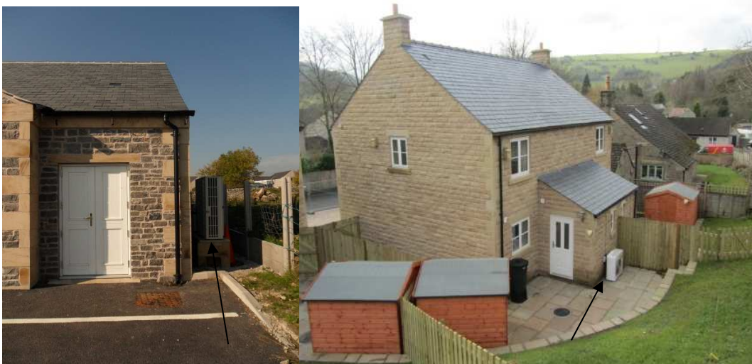
Photo 14. Air source heat pumps at Over Haddon Village Hall and on a new affordable home in Calver
