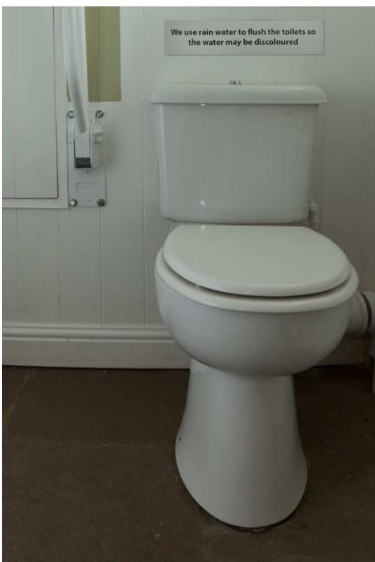
Figure 13 Rainwater harvesting for toilet flushing
