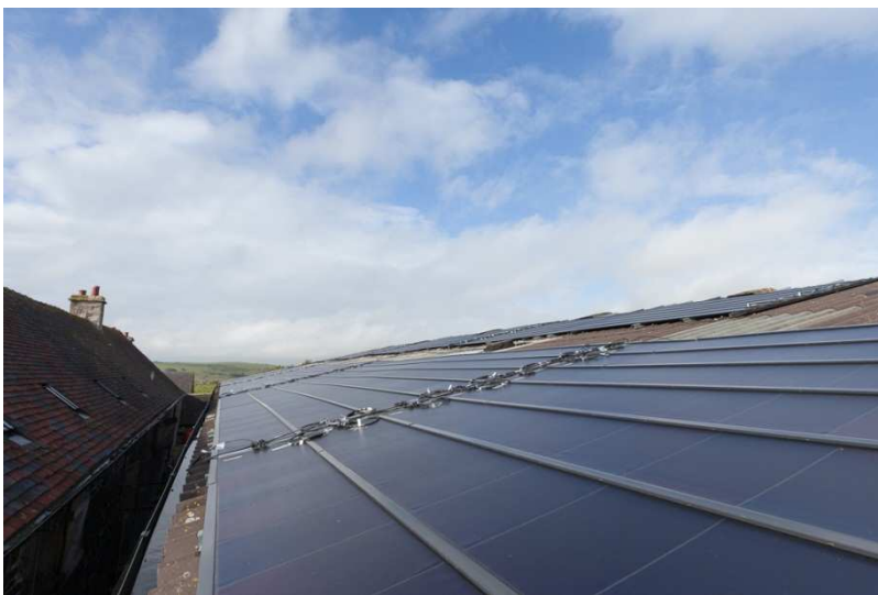
Figure 12 Photovoltaic sheeting installed on portal framed building. Location of installation minimises impact on landscape surroundings
