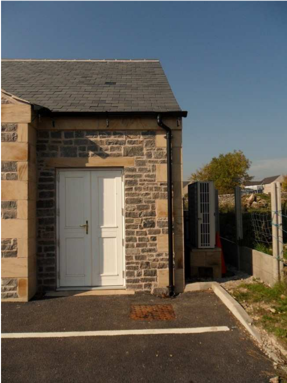
Figure 4 Air Source Heat Pump
