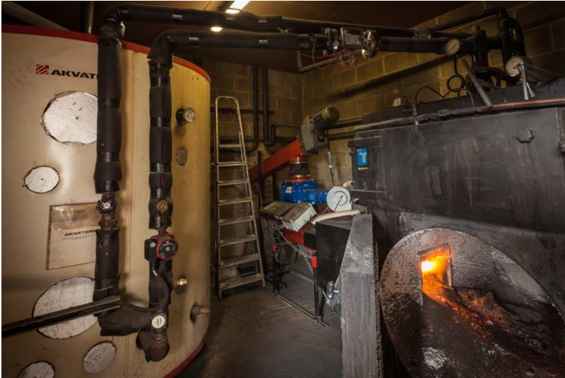
Figure 10 Wood gasification heating system and water storage cylinder
