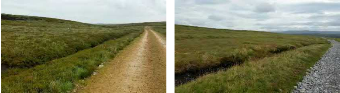
Figure 4.9 Stone tracks with drainage channels running parallel to the track on the upslope side.
