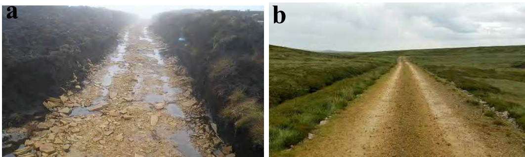
Figure 2.3 a-b a) Example of a ‘cut and fill’ road where the peat has been excavated and aggregate placed along the base of the trench to form the travelling surface. Photo Courtesy of North Pennines AONB. b) Example of floating road on blanket peat where the aggregate is placed on top of the peat surface.
