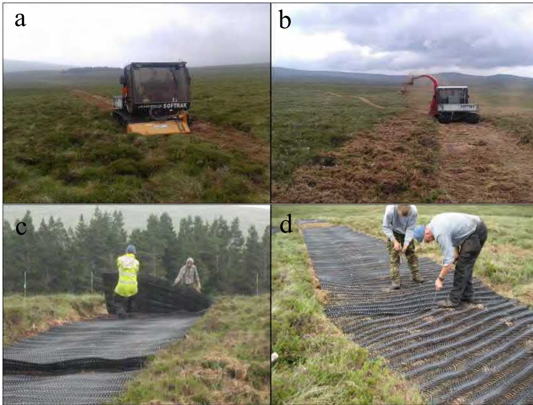
Figure 3.8 a-d a) Cutting of track route using a SOFTRAK with mower attachments, b) Removal of excess cut vegetation along track route using the SOFTRAK with forager attachment, c) Positioning of plastic mesh along route, and d) pinning of track route into place. Photos a) and b) courtesy of Alistair Lockett (North Pennines AONB Partnership).
