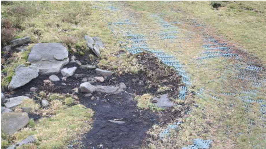
Photo 5 – looking east along mesh track – at base of incline. Erosion by vehicle turning – mesh damaged and breaking up. Limited vegetation establishment.
