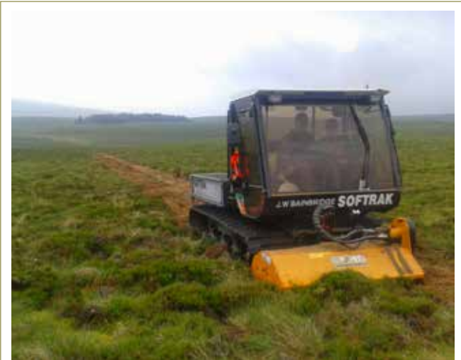
Fig 3. Route of mesh track was cut.
