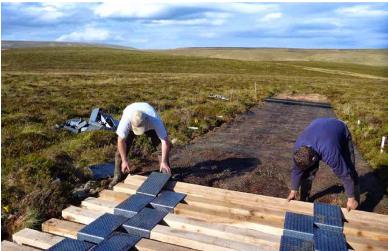
Fig 7. Wooden track being laid after vegetation was cut and removed and plastic grid rolled out.
