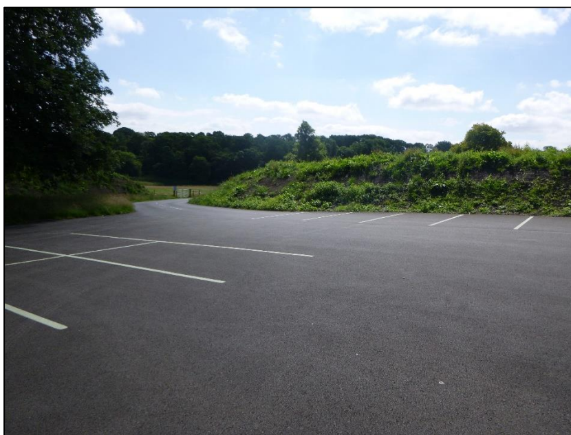
Photograph 7 showing the bare ground at the car park
