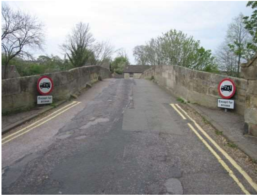
Figure 10.13 – Double yellow lines at the approach to Baslow Bridge
