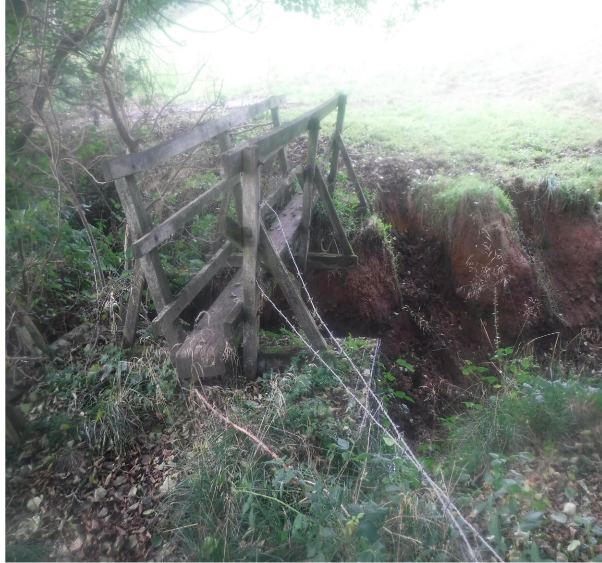
Footbridge losing its footings due to poaching at parish boundary of Kirk Ireton FP 29/Biggin FP 17
