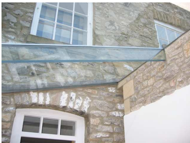
36 This glazed link allowed extension to historic cressbrook mill without harm to the buildings integrity.
